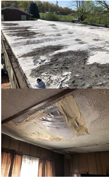
Figure 3. Weatherization Deferral Due to Roof Issues Resulting in Ceiling Damage
